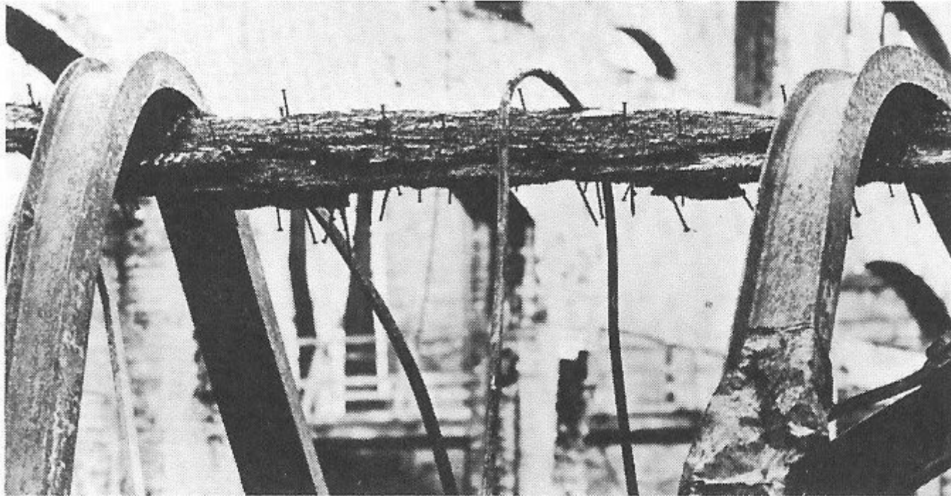
Fig. 20-4. After fire scene. Shows a wood beam supporting twisted steel I-beams. (Forest Products Laboratory)
